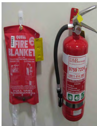
Call Centre extinguishers
