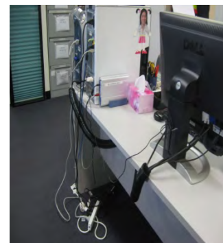
Work station wiring
