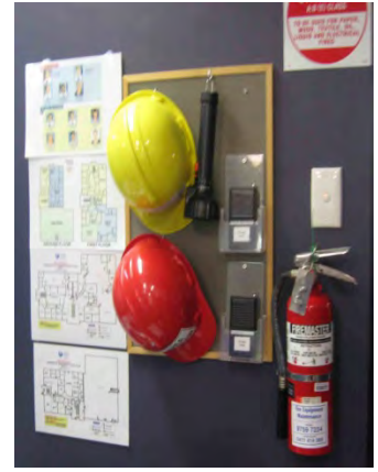
Fire Warden equipment
